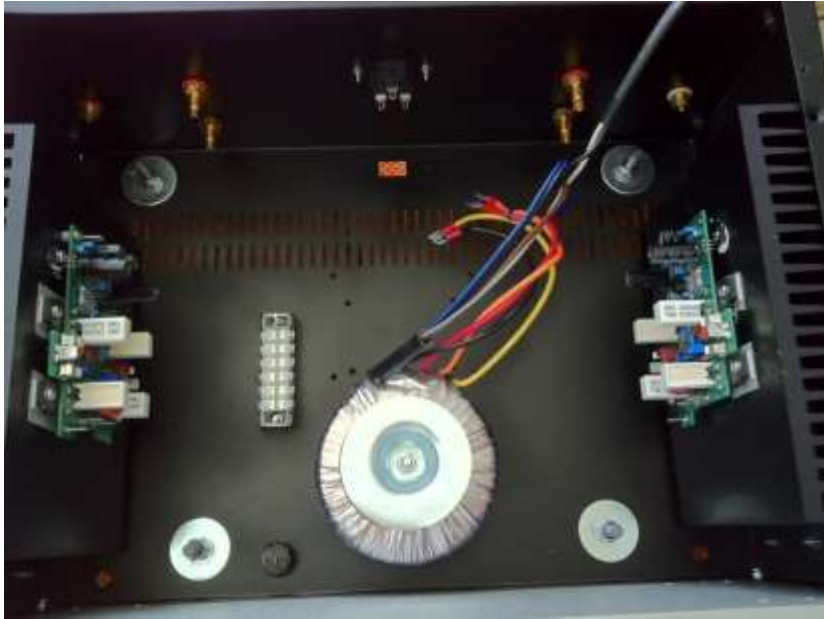
Photo 6 - General Arrangement of Components – the ON/OFF Switch is Located at the Bottom Left of Center (this example is of the first of two sx-Amps built)
